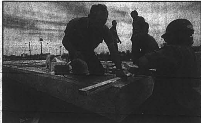
Employees of the Water, Electric and Street Department of Russell construct a platform Thursday afternoon to be used this morning for Dole's pancake breakfast.
